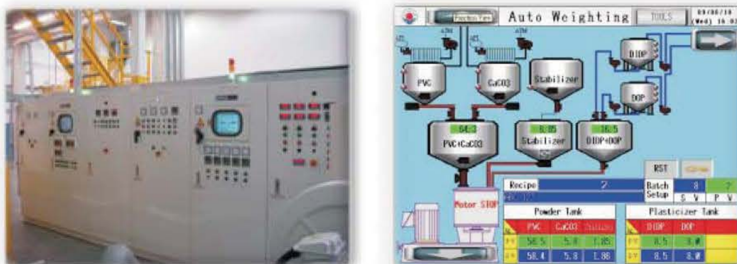
PLC Control & Auto Weighting Touch Screen
