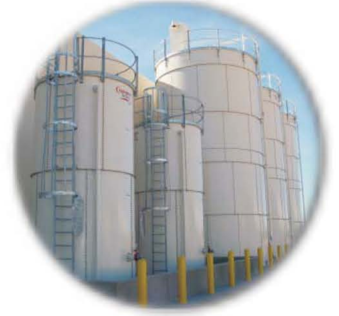
Liquid Storage Unit
